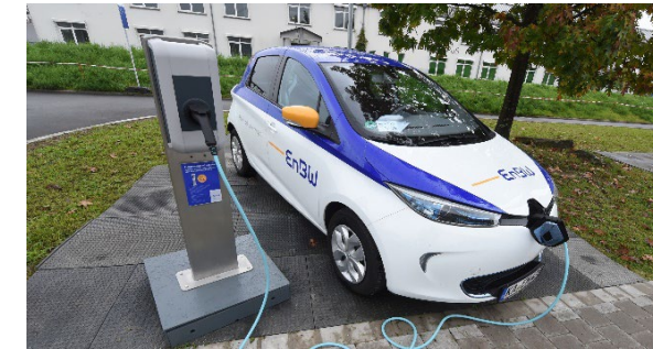
E-mobility charging infrastructure
