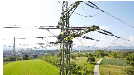
Electricity distribution infrastructure
