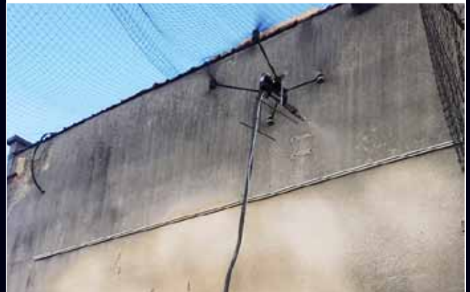
Spraying ► Construction ► Mortar coatings Ornamental coating with clay-based mortars in Brussels (Belgium) MuDD Architects, France
