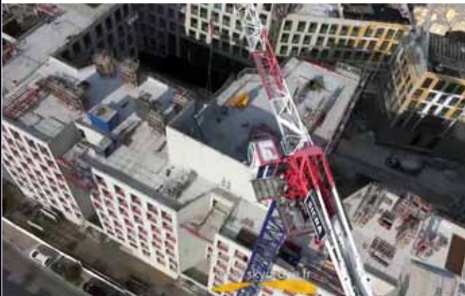
Spotting ▶ Construction & Real Estate ▶ Construction errors Skydrone, France
