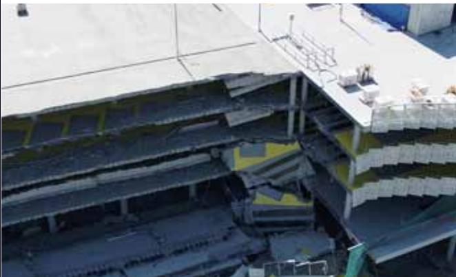
Inspection ▶ Insurance ▶ Post-accident/disaster ▶ Building collapse Inspection after collapse of parking garage at Eindhoven airport Euro Drone Inspections, The Netherlands
