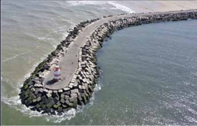
Surveying ► Maintenance ► Breakwater repair assessment The port of Scheveningen, The Hague - CDR International, The Netherlands
