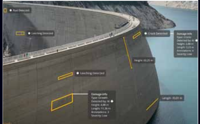
Spotting ► Maintenance ► Cracks ► Dams EasyInspect, Denmark
