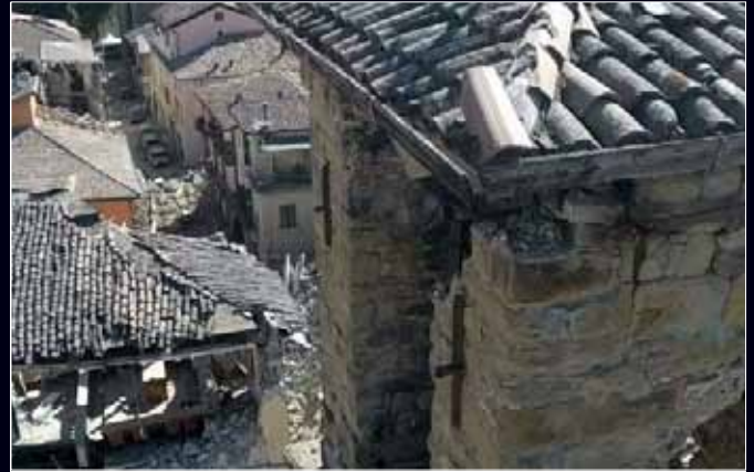
Inspection ▶ Heritage Sites & Historical monuments ▶ Post disaster 2016 Earthquake - CNVVF National Fire & Rescue Services, Italy
