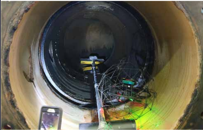
Inspection ► Maintenance ► Infrastructure ► Pipelines (interior) Inspection of a pipe section - PowerFox, Australia
